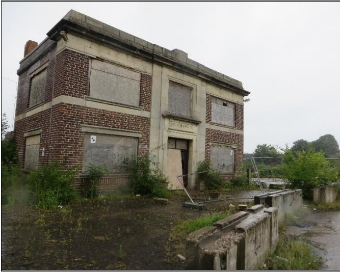
Part of a derelict building located in the north of the site
