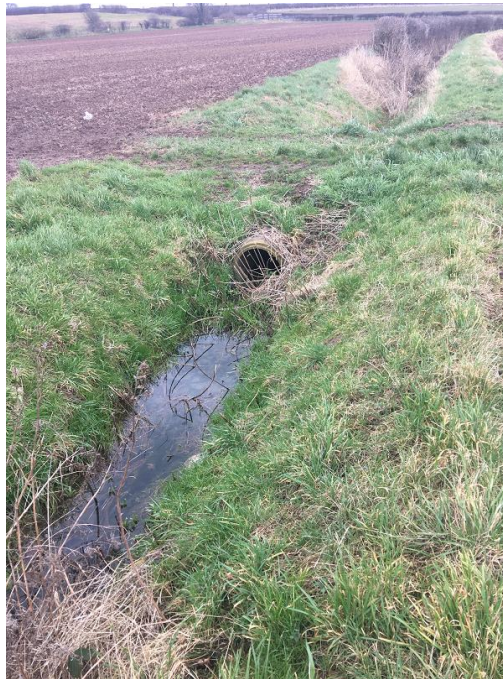
Figure 2-2: Piped culvert to allow continuation of flows for the central watercourse flowing across the site.
