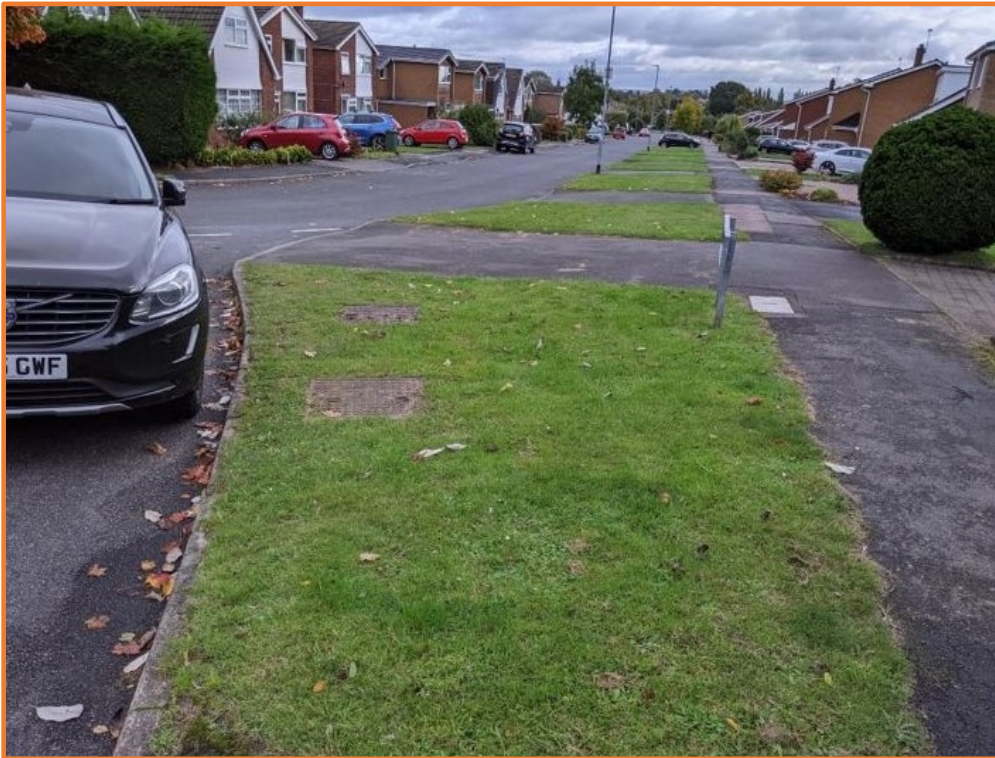
Photo of adopted drainage network in Leconfield Road.
