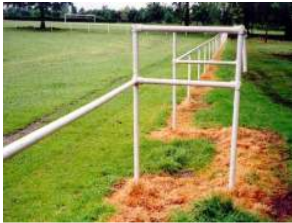
This shows an unacceptable obstacle spraying and strimming on a volume / amenity site within sporting facilities.
